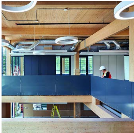
Canadian Nuclear Laboratories asked HDR to revitalise its site at Chalk River, Ontario
